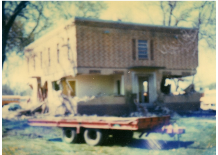
Above: The razing of the 1931 jail on April 10, 1986. According to The Coffey County Today April 11, 1986, issue of the newspaper, "The plan was to let the top story fall after moving most of the support but the old building proved tougher than some thought."
