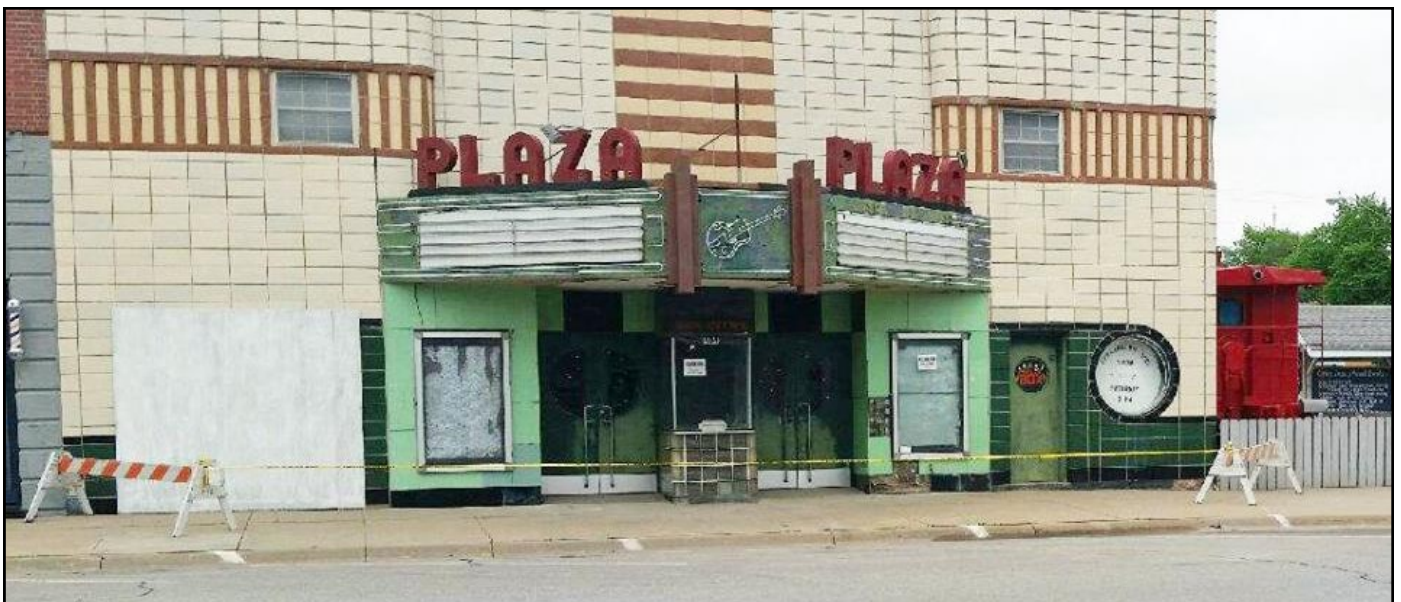
Above: The current condition of the Plaza theatre building. A barricade had been set up in the front of the building in case tiles fall off and a board covers up a hole in the building when a car drove through it on December 2, 2014.
